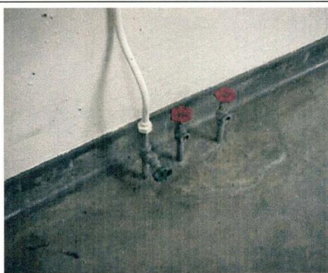
Figure 2 W-K Taps for Kaplan Unit
